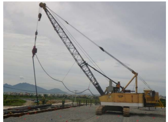
Moving treatment system equipment to top of containment structure (Photo: CDM Smith)
